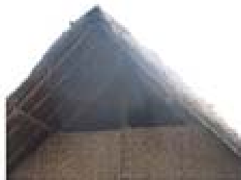
Figure 6: The holes in the gable end of roof
